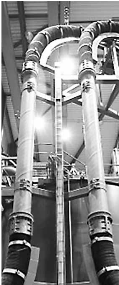
Picture 1: Material handling hose and rubber lined steel pipe
