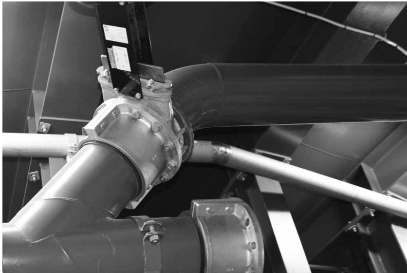
Shut off valve for slurry pump line with K45 branch pipe
