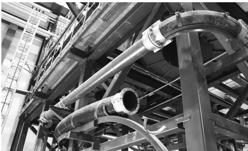
Picture 3: Material handling hose, rubber lined steel pipe, 3x90 degree bend and support clamps
